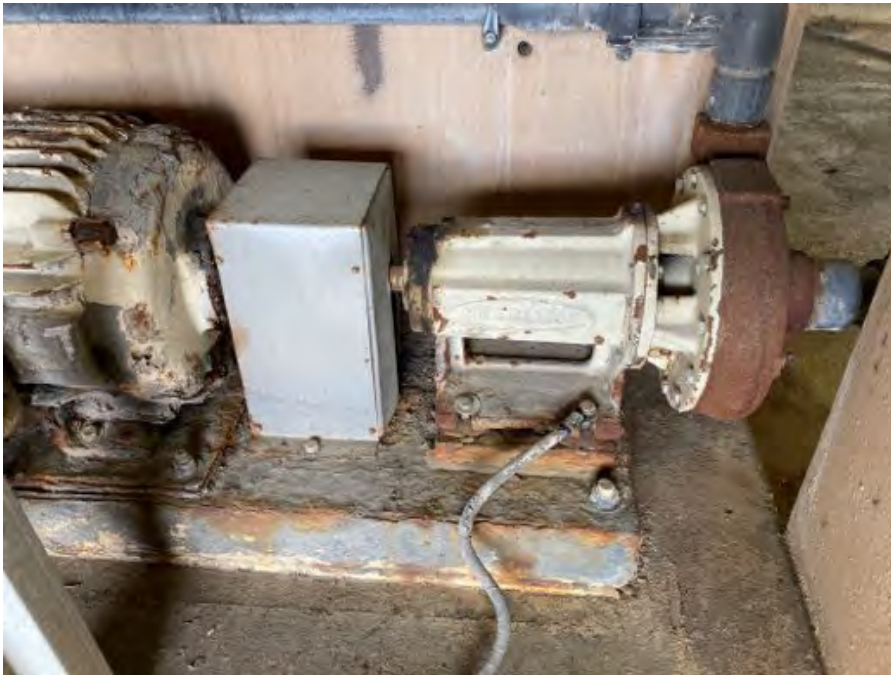
Figure 6-16. Wash Water Pump
