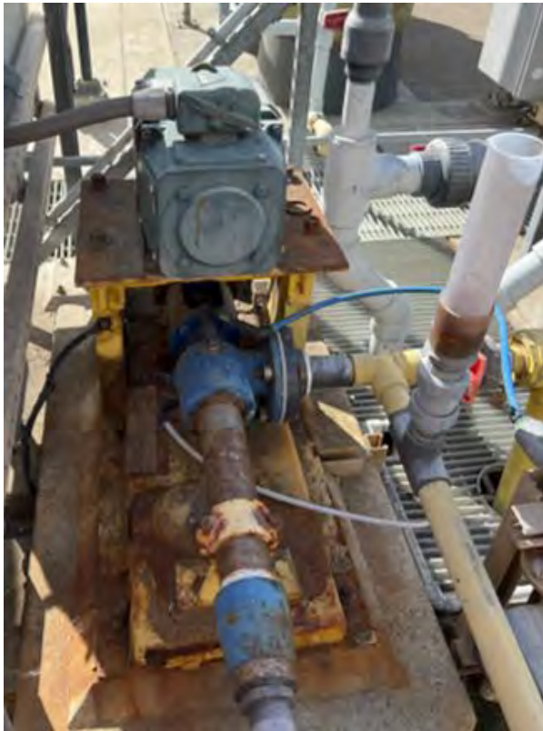
Figure 6-17. Polymer Feed Pump
