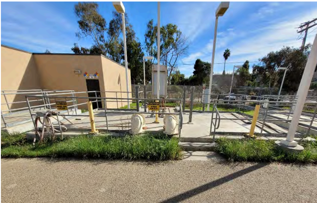
Figure 4-4. Hollister Street Pump Station Wet Well
