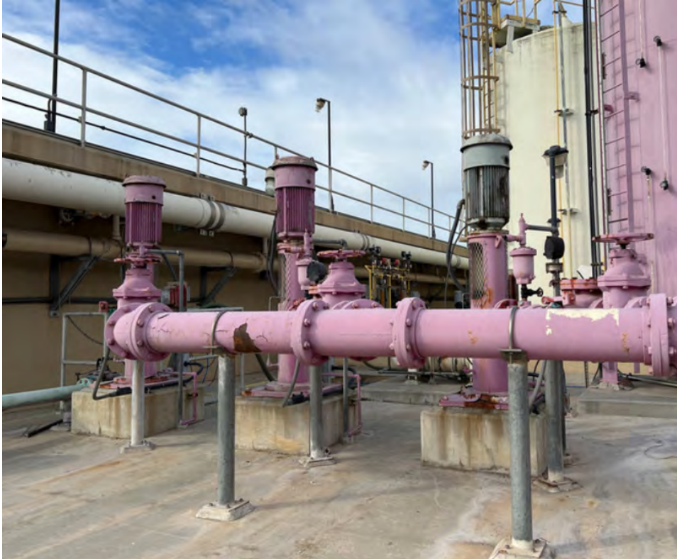
Figure 7-20. Pumping Area for NPW Pump Station No. 1
