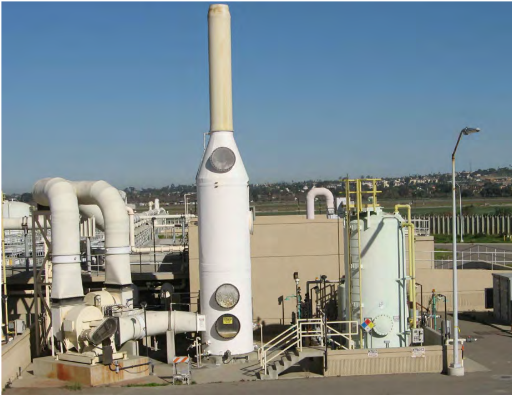
Figure 7-6. Primary Sedimentation Tank Odor Reduction Station
