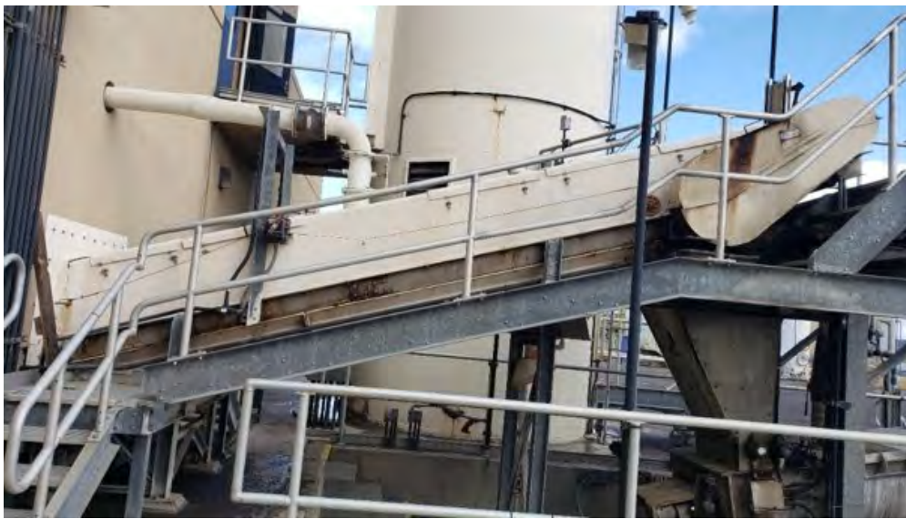
Figure 6-18. BFP Conveyor No. 1B
