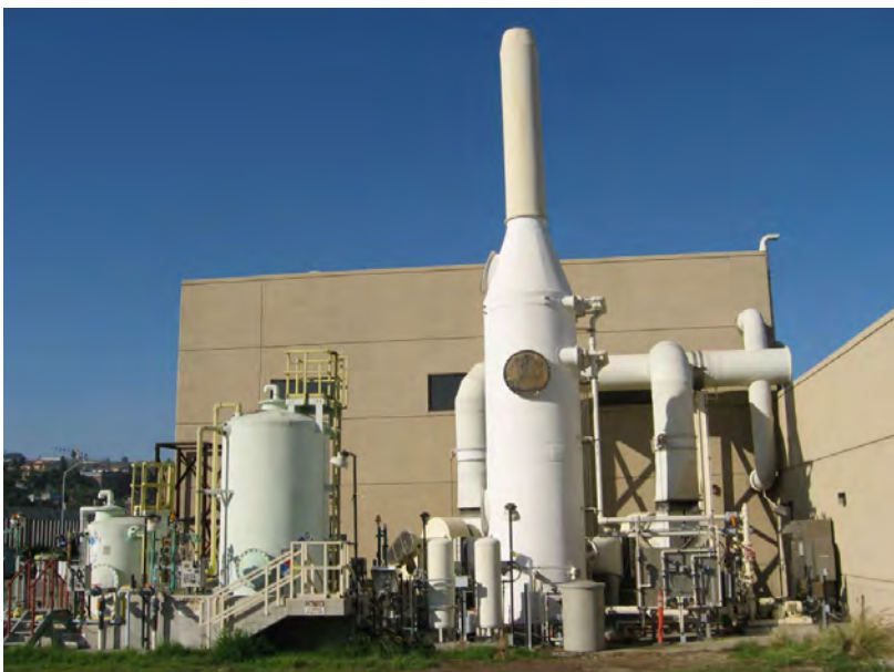
Figure 7-1. Headworks Odor Reduction Station
