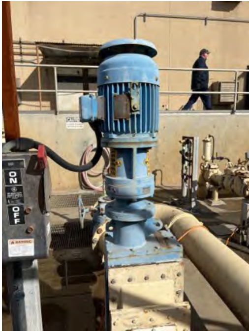
Figure 6-13. Sludge Feed Grinder
