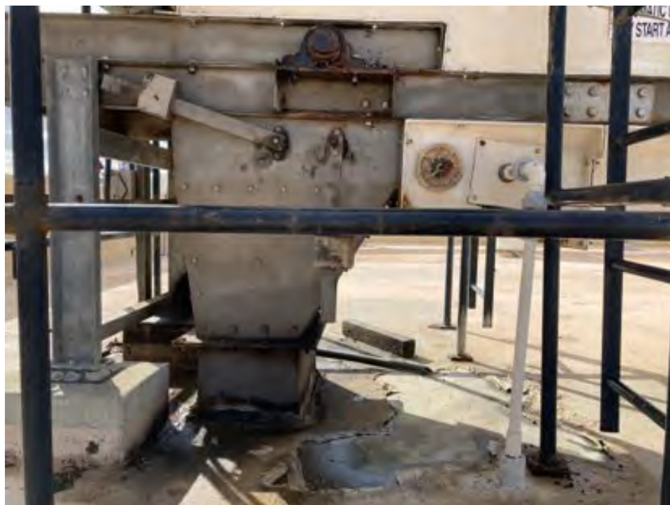
Figure 6-24. Truck Loading Conveyor Roof Discharge
