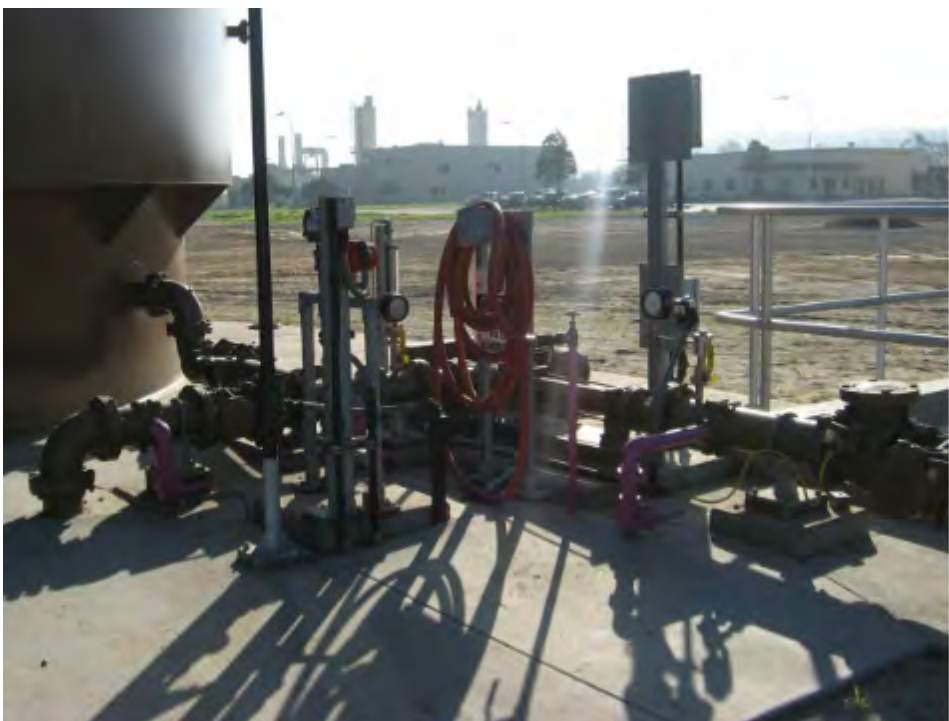
Figure 6-3. TWAS Pump and Metering System
