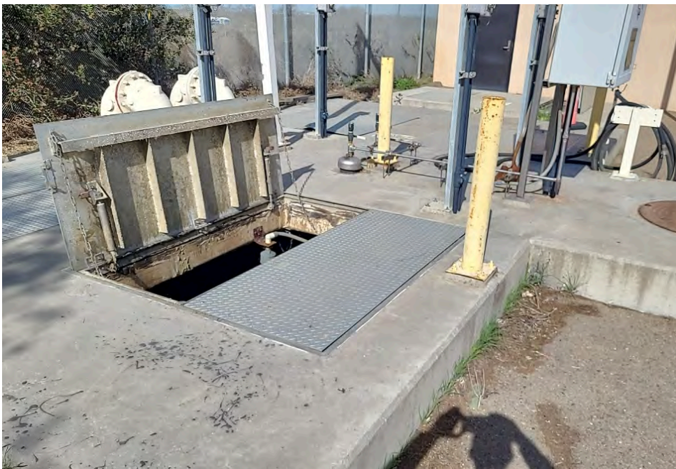
Figure 4-2. Goat Canyon Pump Station Wet Well
