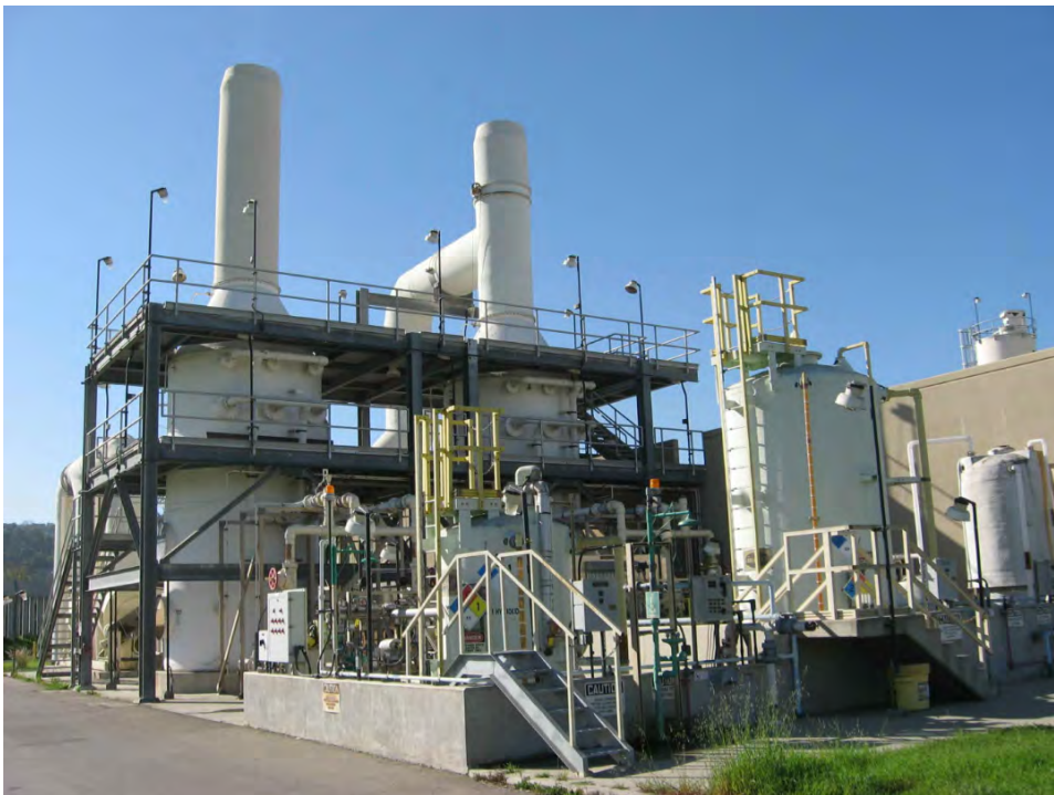
Figure 7-9. Solids Processing Odor Reduction Station
