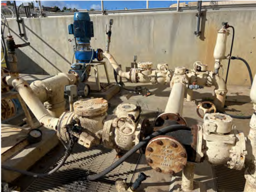
Figure 6-14. Sludge Feed Pump Station
