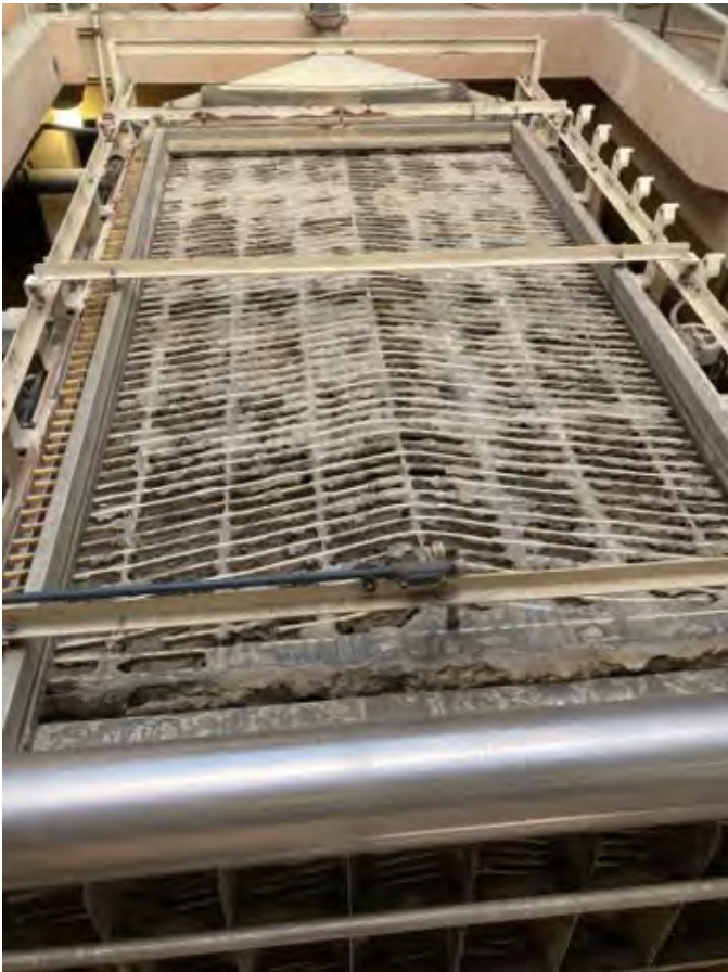
Figure 6-15. Existing BFP (from top)
