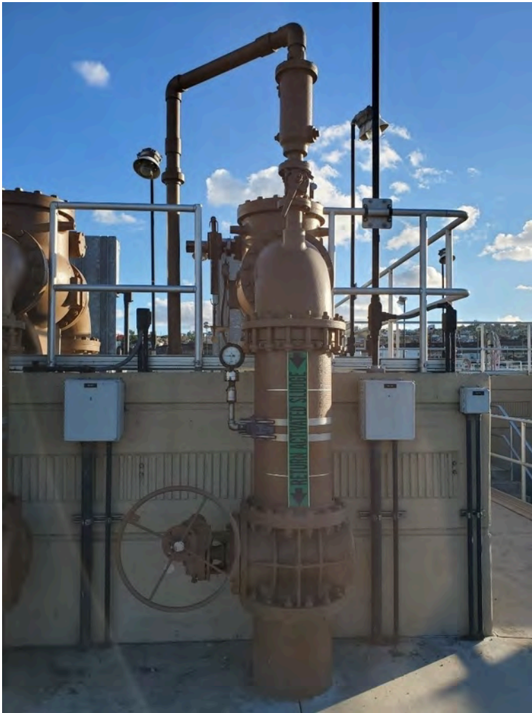
Figure 5-22. Top Deck of the RAS Pump Station
