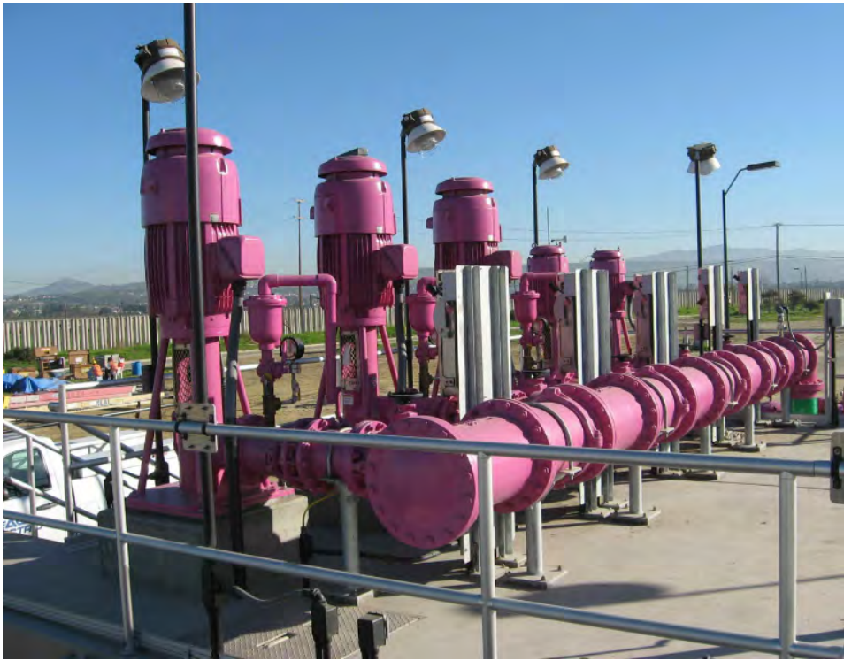
Figure 7-21. Pumping Area for Non-Potable Water Pump Station No. 2
